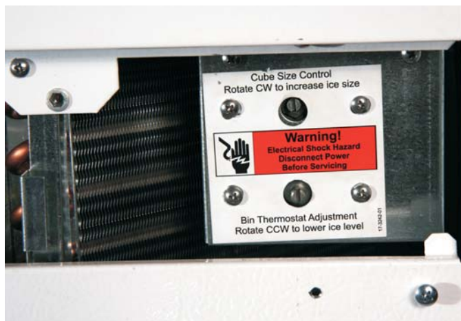
Condenser and Bin Thermostat
